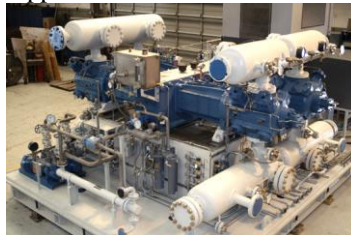
Figure 1 An example of a medium size horizontal-type reciprocating compressor for a process application. Suction pulsation bottles are installed above the cylinders. Discharge pulsation bottles are installed under the cylinders.
