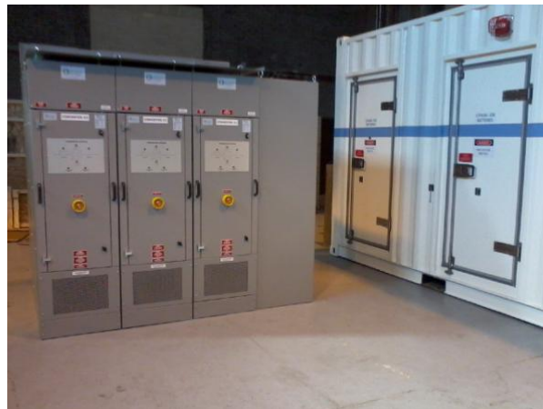
Figure 2. Site View of the Energy Storage System and Battery Container
