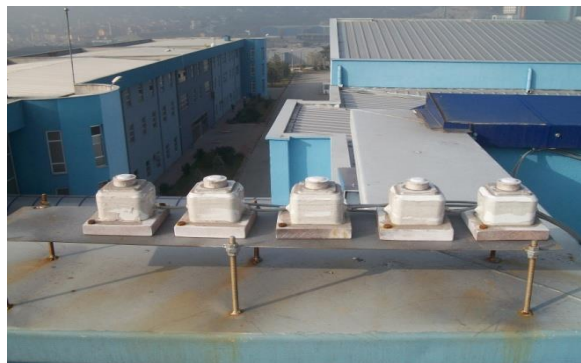
Figure 2. Horizontally placed pyranometers.
